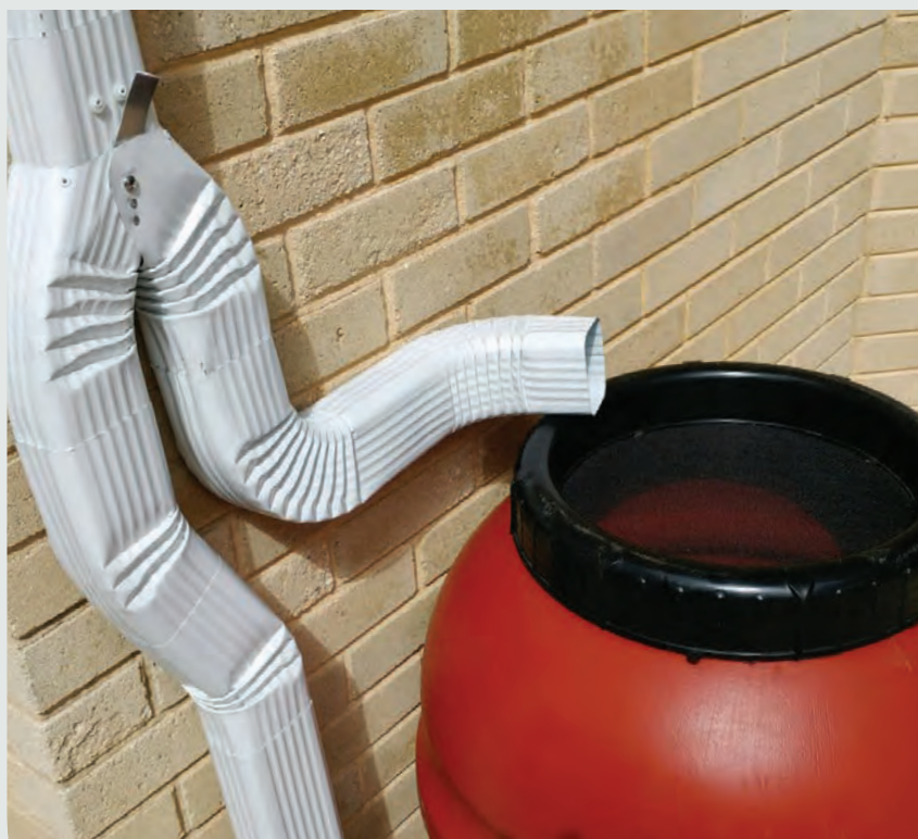
This diverter has a flap at the top, which can be switched to allow flow to go into the rain barrel (right downspout) or flow through the downspout onto the ground (left downspout).
