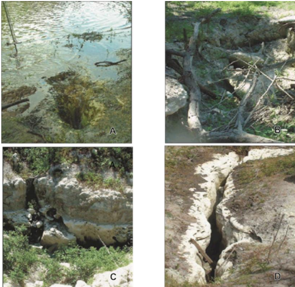
Figure 2-21. Prominent karst features in the Upper Peace River basin observed during dry river conditions in mid-May 2002. Features includes: (A) Fricano fracture, (B) Midway sink, (C) Dover sink, and (D) the crevasses. These features were documented during a USGS study in cooperation with the District. Adapted from Knochenmus (2004).
