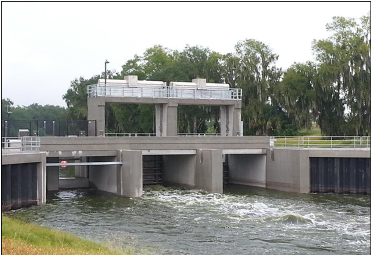
Figure 2-40. Downstream view of the Lake Hancock P-11 control structure, showing two weir gates in the leftmost bay (one partially open and one closed) and roller gates in the other two bays. Adopted from Yang et al. (2020).
