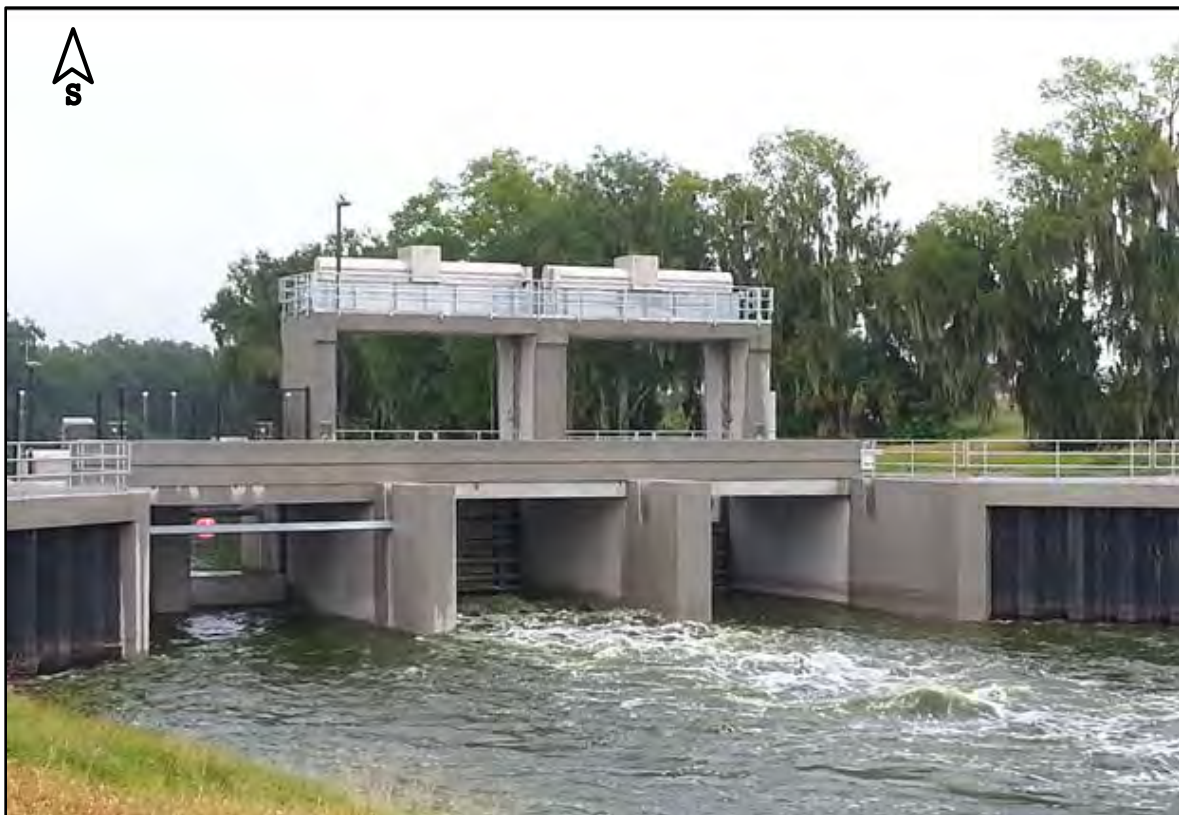
Figure 5. Downstream side of the Lake Hancock's P-11 control structure showing two weir gates in the westernmost bay on the left (one is partially open and the other is closed) and roller gates in the other two bays
