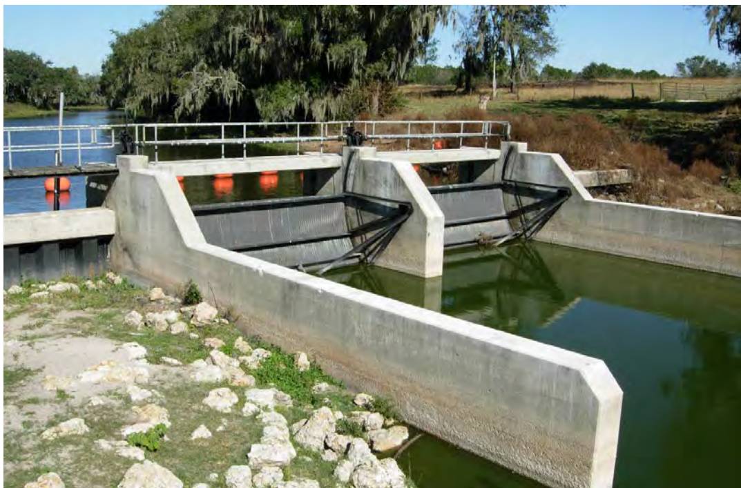
Figure 4. Downstream side of the former P-11 control structure showing two metal radial gates and the concrete-capped, sheet-pile wall
