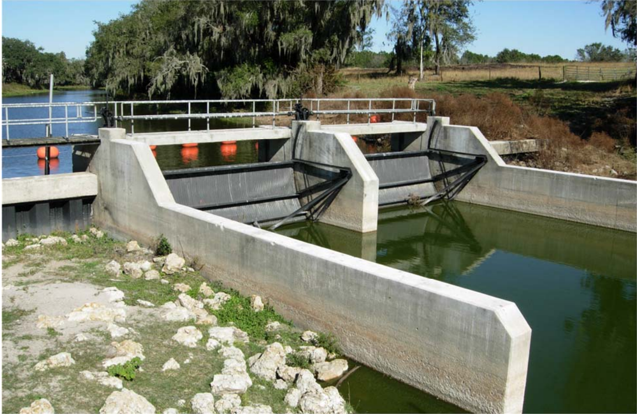
Figure 4. Downstream side of the former P-11 control structure showing two metal radial gates and the concrete-capped, sheet-pile wall
