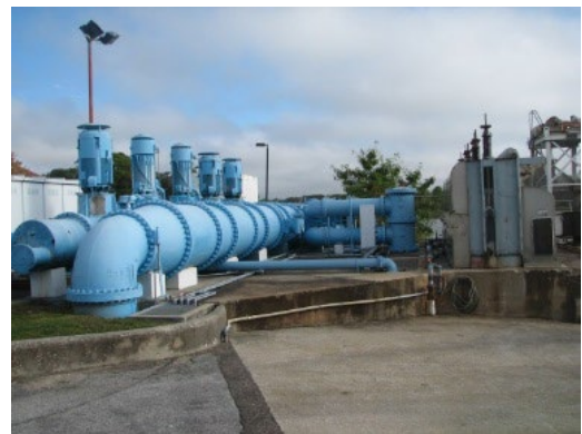
Potable water pumping station
