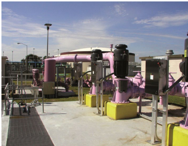
Reclaimed water facility in Hillsborough County
