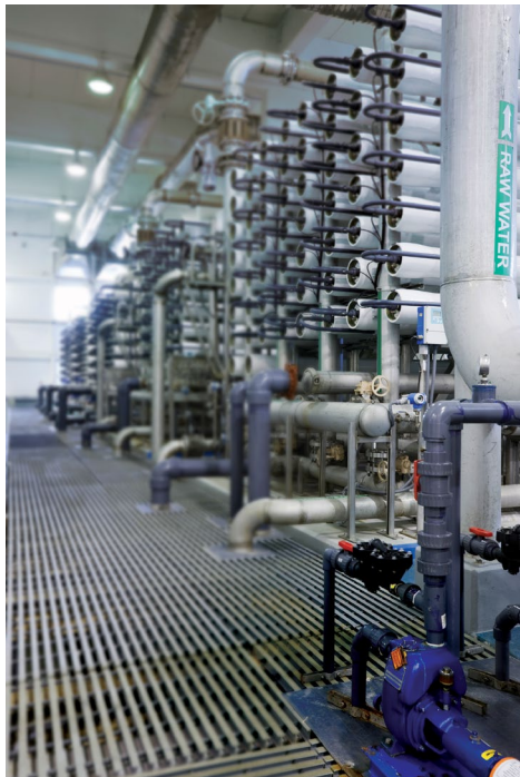
Tampa Bay Water desalination facility
