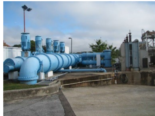
Potable water pumping station
