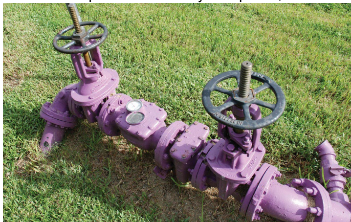
Reclaimed water pipe
