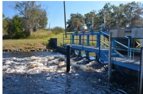
Control structure at Tsala-Apopka Outfall
