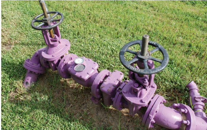
Reclaimed water pipe
