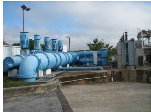
Potable water pumping station
