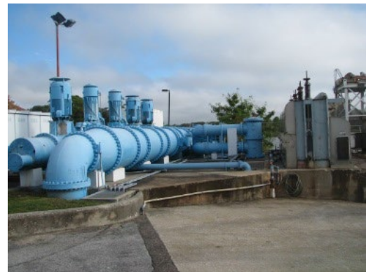
Potable water pumping station
