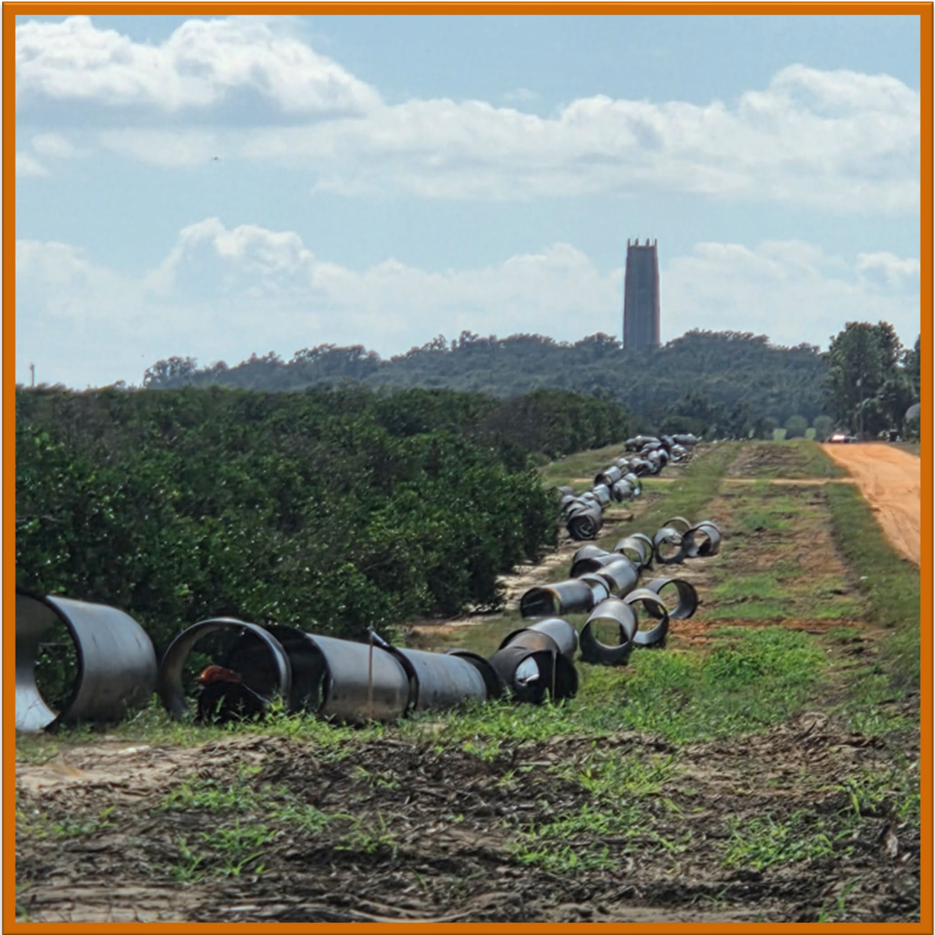
Polk Regional Water Transmission, 30" ductile iron pipes staged for installation near Bok Tower in Lake Wales.
