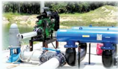
Surface Water Irrigation Pumps and Filters
