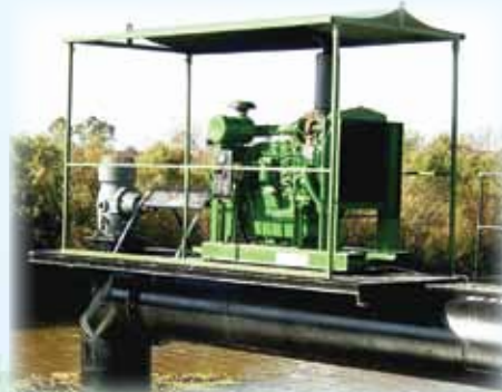
Tailwater Capture and Reuse Pump Stations
