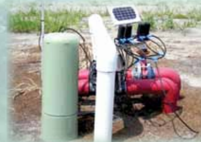
Remote Irrigation Zone Controls and Soil Moisture and Climate Sensor Telemetry
