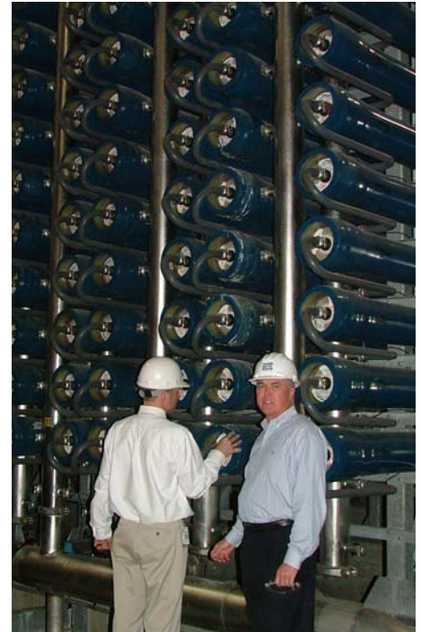
CLA staff recently facilitated a tour of Tampa Bay Water’s Desalination Plant in Apollo Beach for State Representative Ron Reagan. The District is a partner in the plant, which, when operational, will be the largest desalination facility in the United States.
