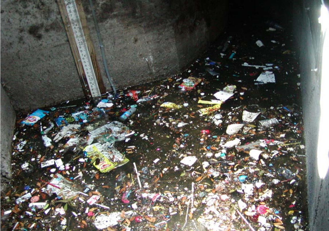
Entrance to CDS unit showing staff gauge and trash during base flow conditions. The diversion weir is off to the right.
