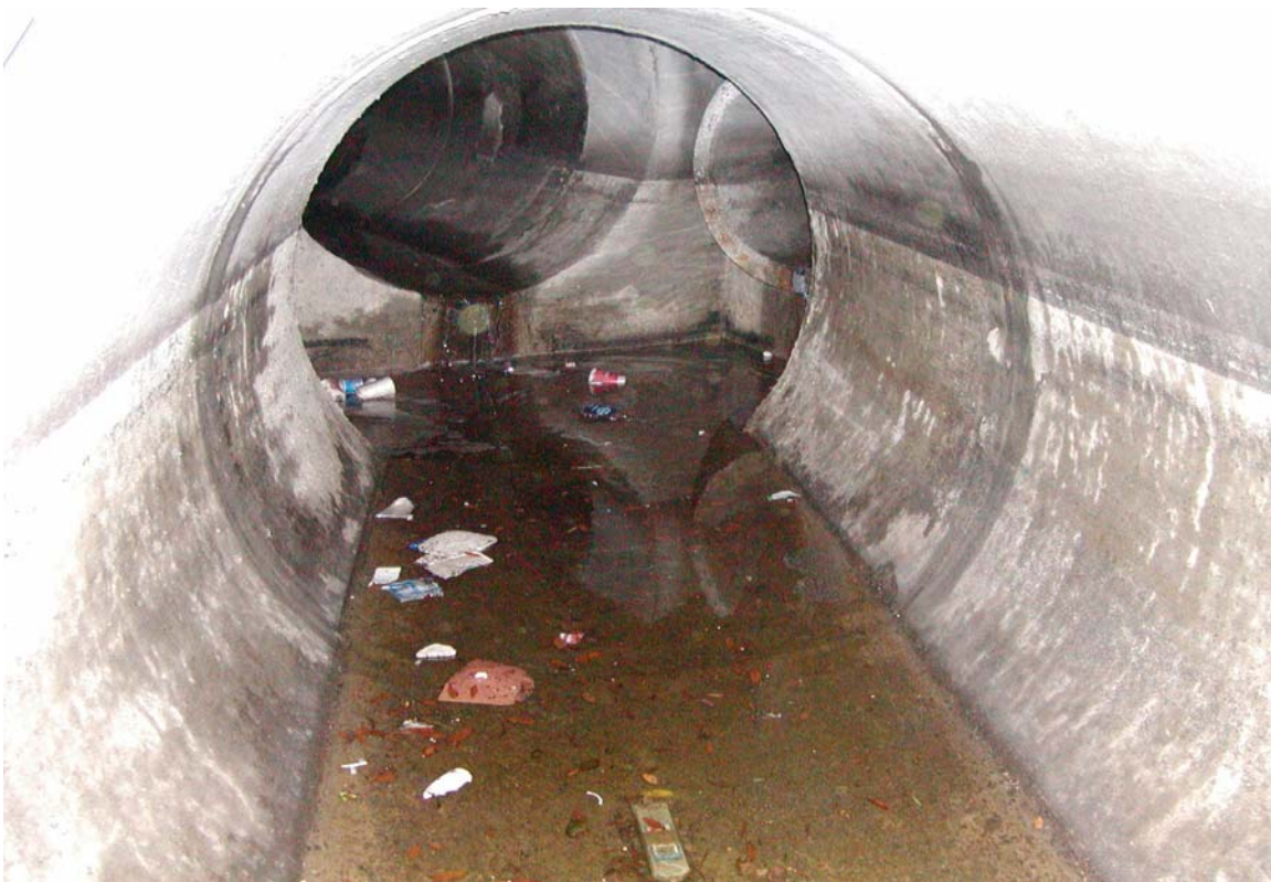
Looking upstream of the CDS unit where three pipes join together.
