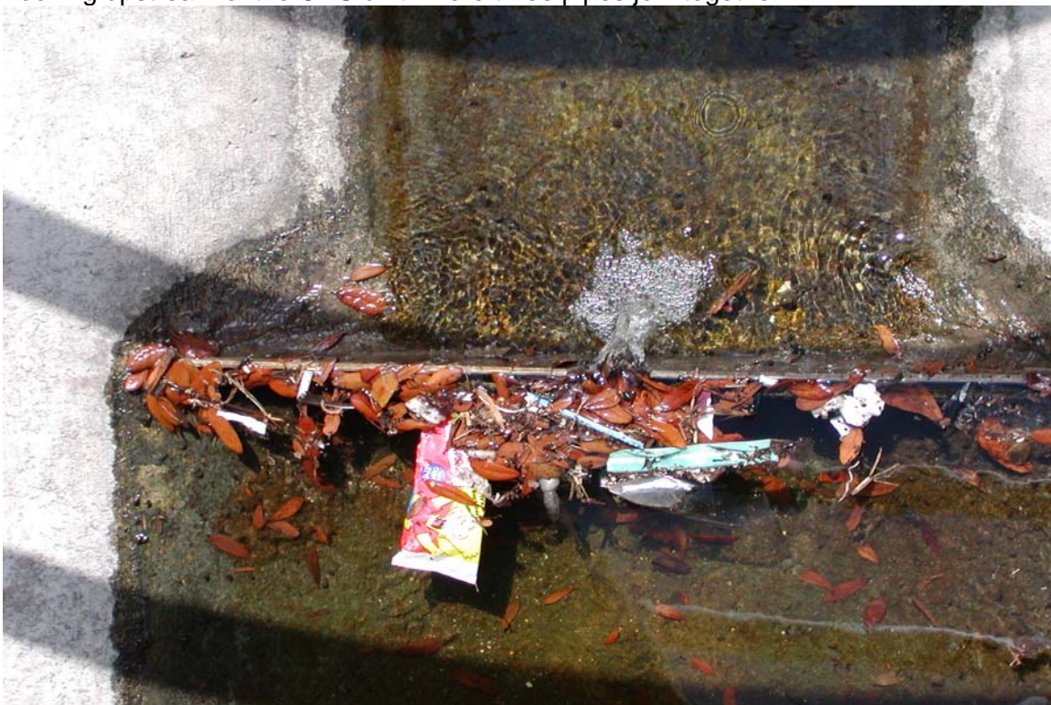
Looking down at base flow weir showing debris backing up water & creating measurement problems.
