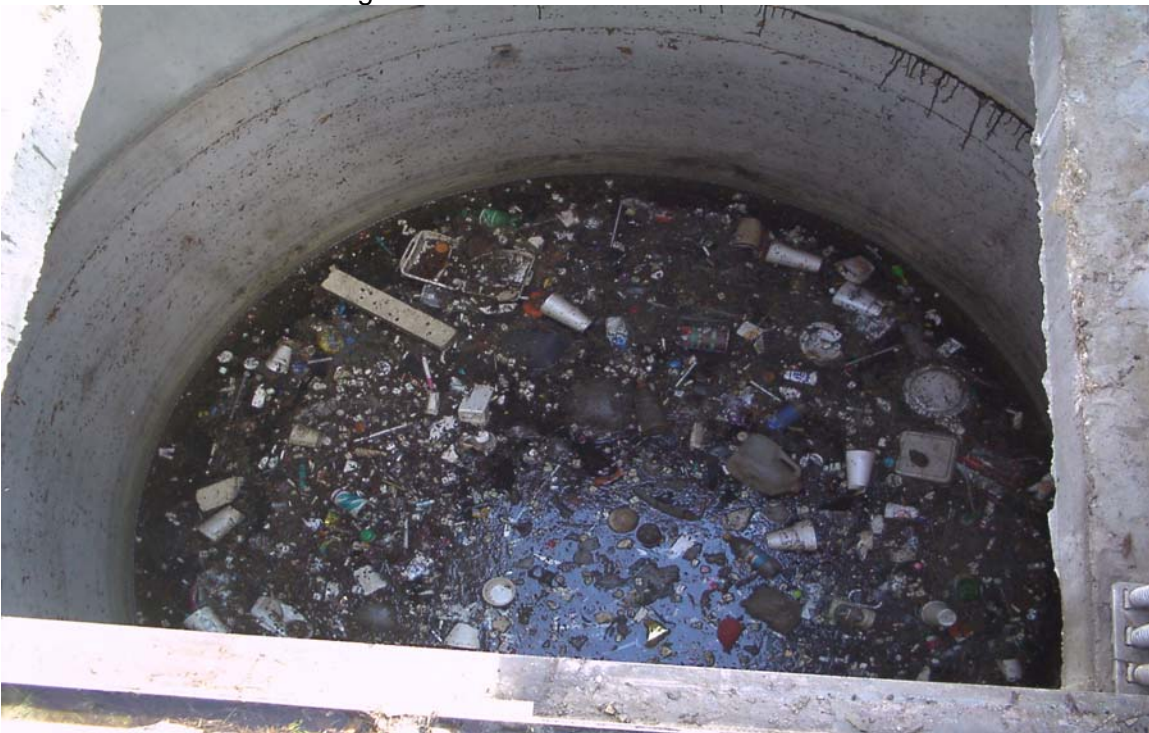
Looking down into the CDS unit from the top.
