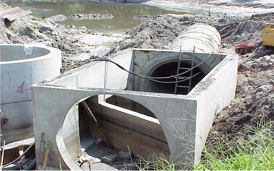
Installation showing CDS to left, diversion weir in collection chamber of pipe
