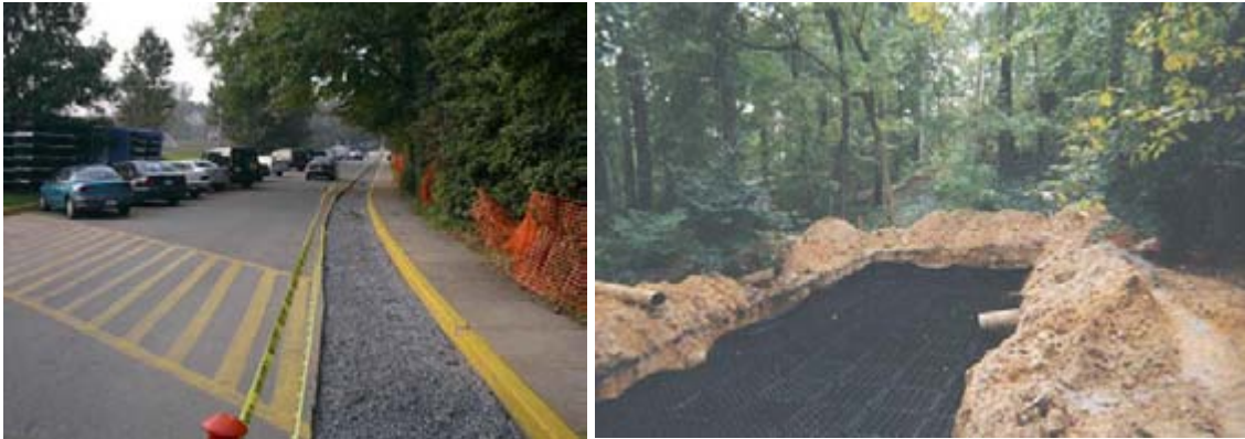
Infiltration Trench in Roadway and “Rainstore” Infiltration Bed at Washington National Cathedral
